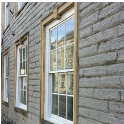
Insulated DPC is not visible in typical sash window re-installation
