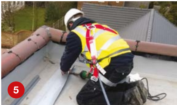
5 Hot-Weld the membrane strap which should be 150mm in width to seal over the fixing line, taking pressure off the existing membrane
