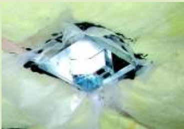
Overlapping of the air barrier, together with caulking around this ceiling air vent, helps to prevent air leakage through the building envelope.
