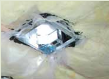
Overlapping of the air barrier, together with caulking around this ceiling air vent, helps to prevent air leakage through the building envelope.
