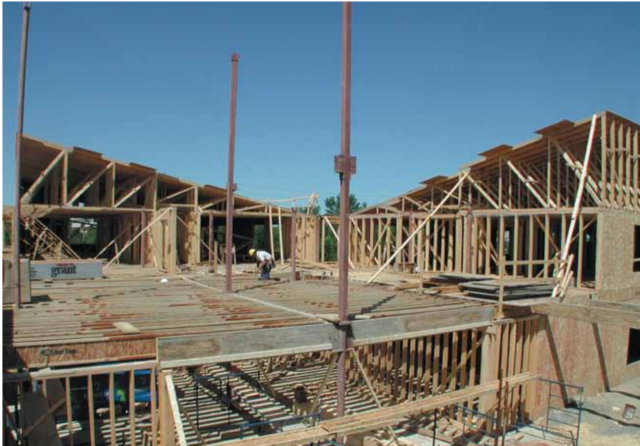
PHOTO 3: Numerous types of light wood-frame building systems are available to maximize fire safety and minimize sound transmission.
