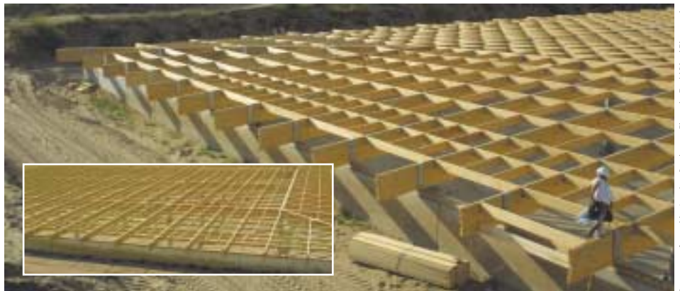
Glulam Yellow cedar beams and trusses frame roof over 5.3 hectare water reservoir.
