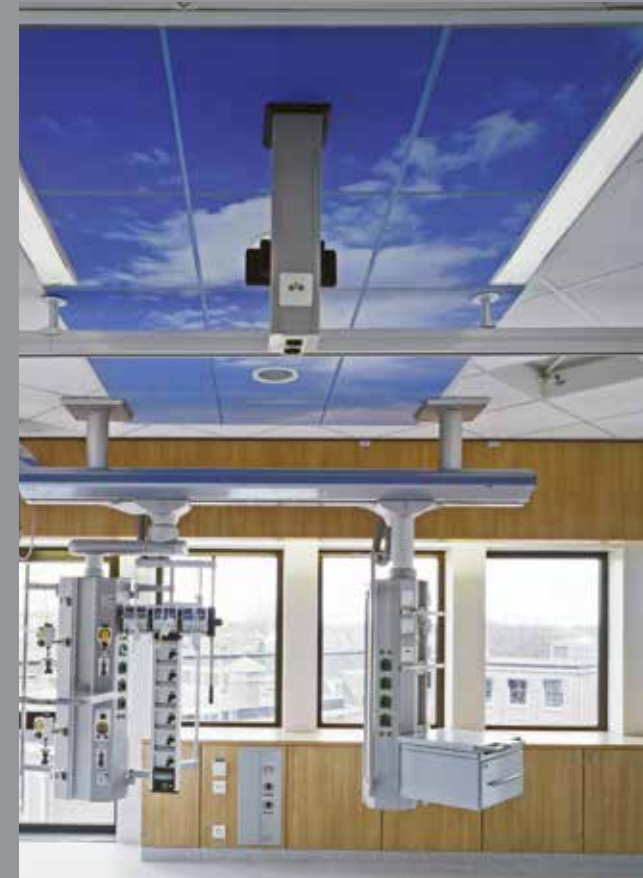
UMCG (NL) Island Ceilings with NEVADA Print Tiles
