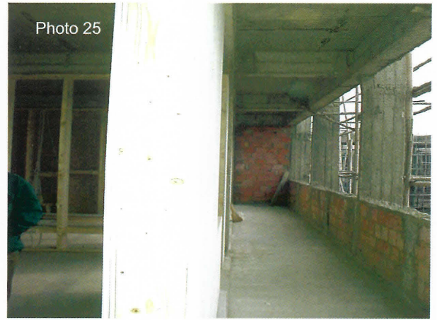
Photo 25 Q-WEB – this is the only original Exterior wood frame wall inset from the building perimeter.
