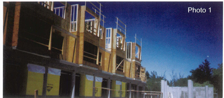
Photo 1 Neale Staniszkis Doll Adams Architects There are many ways to use wood in combination with concrete/masonry. In this case, wood-framed upper storeys are supported by a concrete ground floor.
