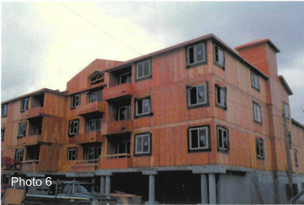
Photo 6 APA-The Engineered Wood Association Hybrid construction combines the best features of concrete and wood construction.
