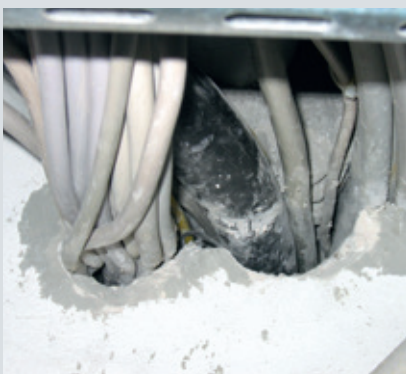
Faulty cable fire stop increases the risk in the event of fire
